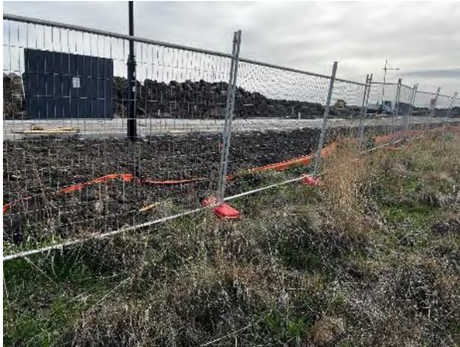
Photo 7: Collapsed and damaged sediment fencing.
