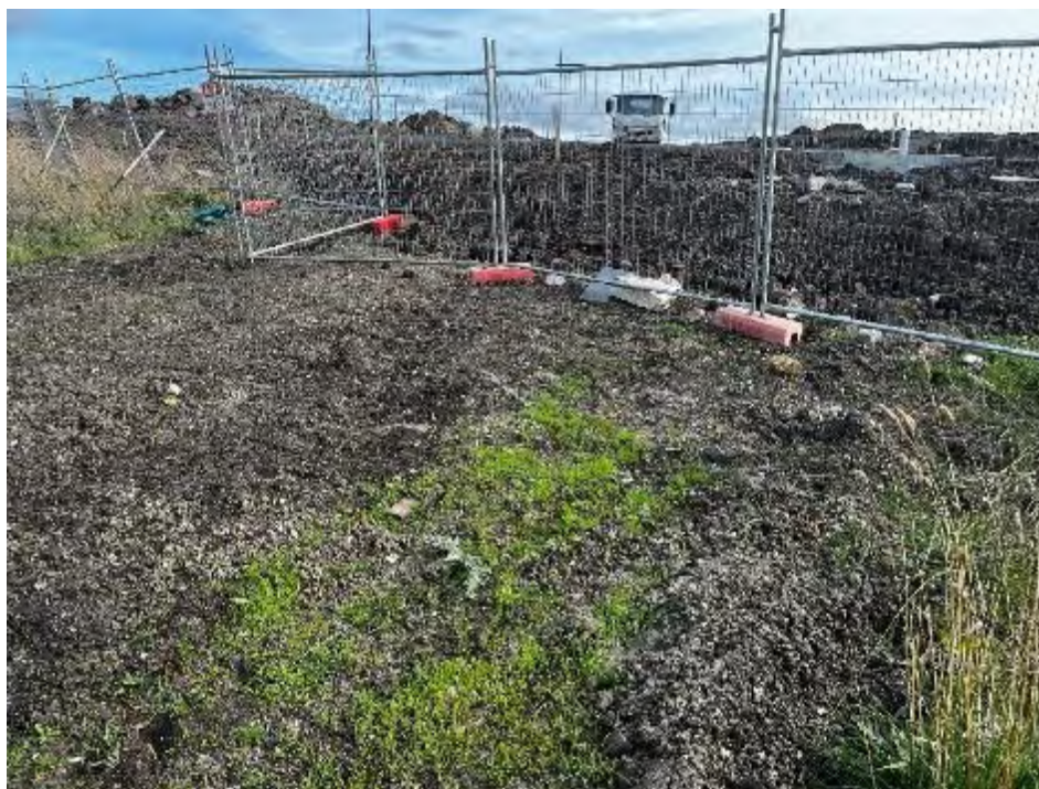
Photo 6: Sediment fencing not present around areas of earthworks
