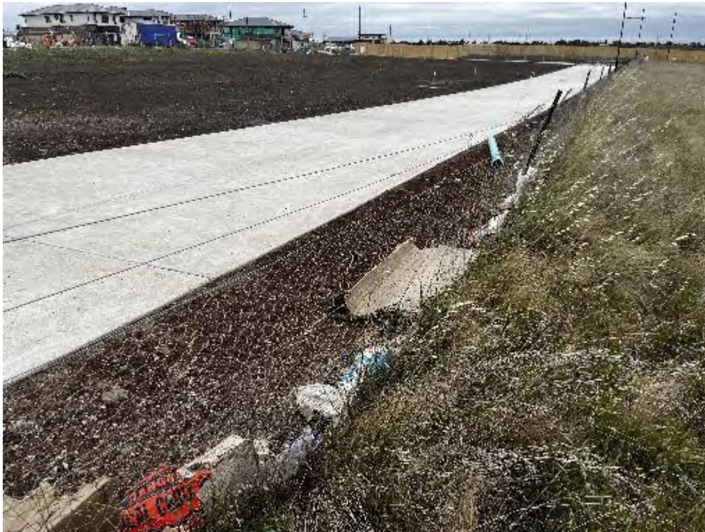
Photo 21: No sediment fencing adjacent areas of construction and earthworks.
