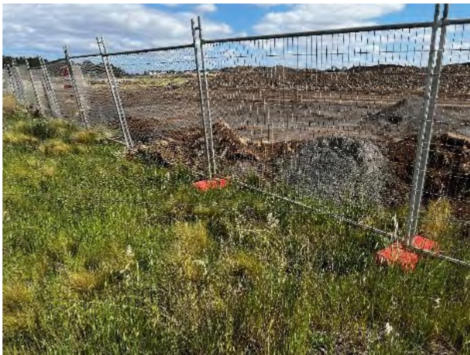
Photo 8: Sediment fencing not present around areas of earthworks
