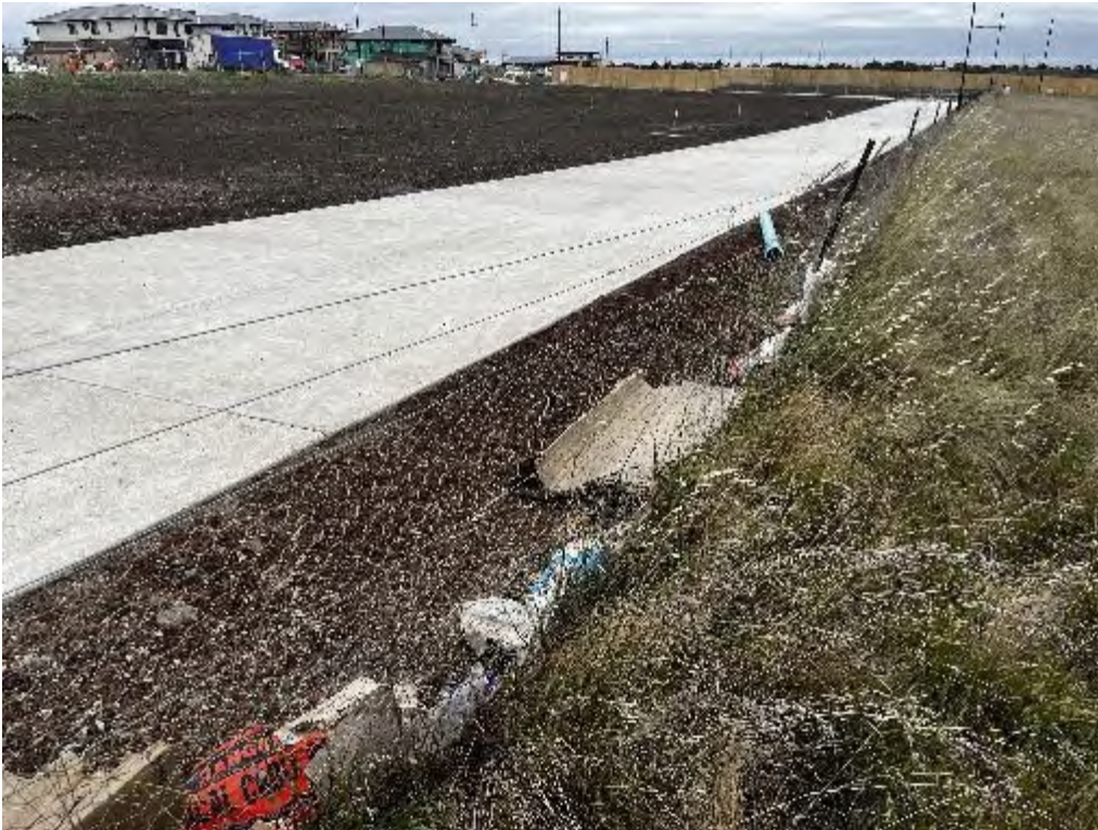
Photo 17: No sediment fencing adjacent areas of construction and earthworks.
