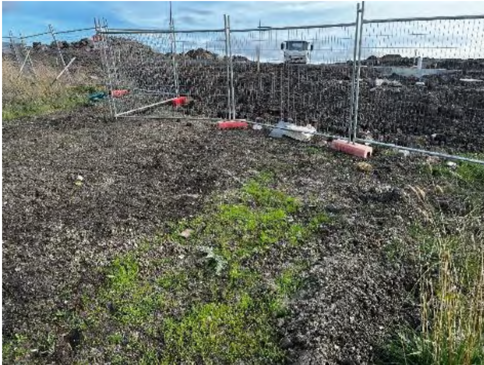
Photo 4: Sediment fencing not present around areas of earthworks
