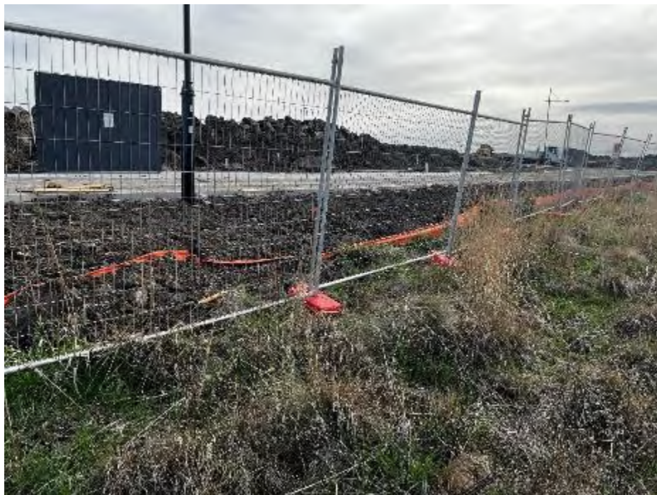
Photo 5: Collapsed and damaged sediment fencing.
